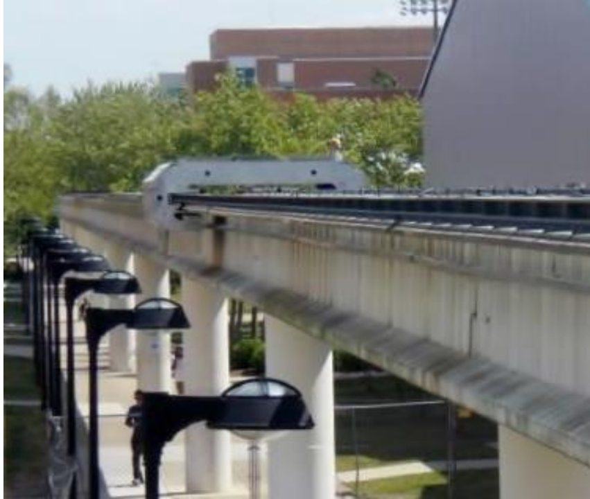
Figure 3a. The M3 system mounted on the guideway at Old Dominion University, Norfolk, Virginia.
